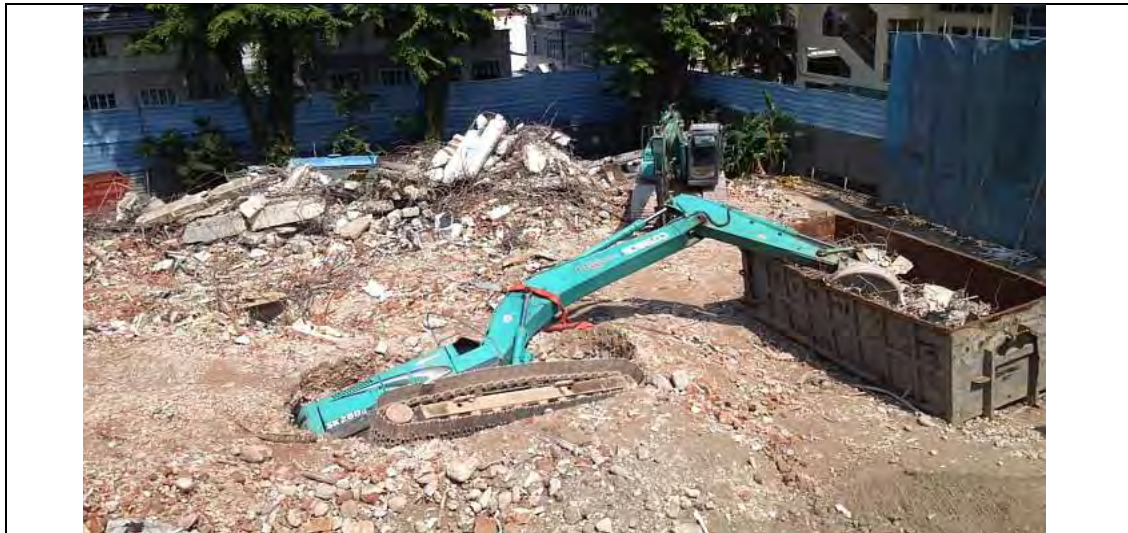
A building was being demolished using an excavator standing on the first floor. The floor collapsed bringing down the building. The excavator fell into the basement and was partially buried by rubble, trapping the operator in the cab. Unfortunately by the time rescuers reached the operator he had died.
