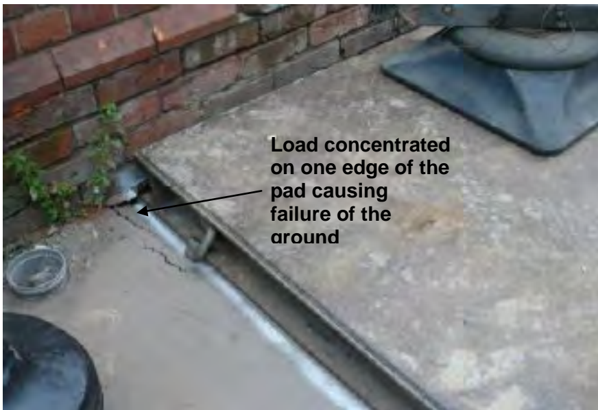
Figure D3 - Example of the Effect of an Offset Outrigger on a Pad
